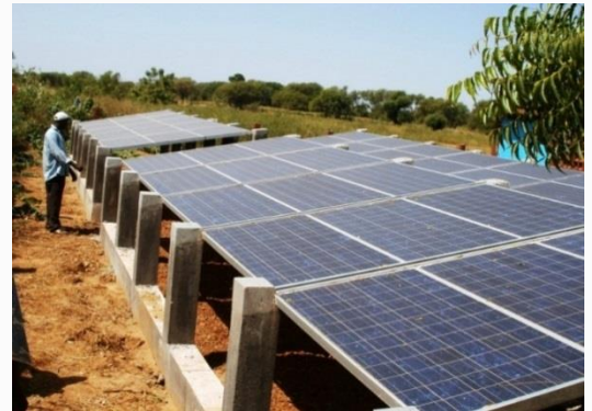
PMRE14 Solar PV Project, Republic of Mali
