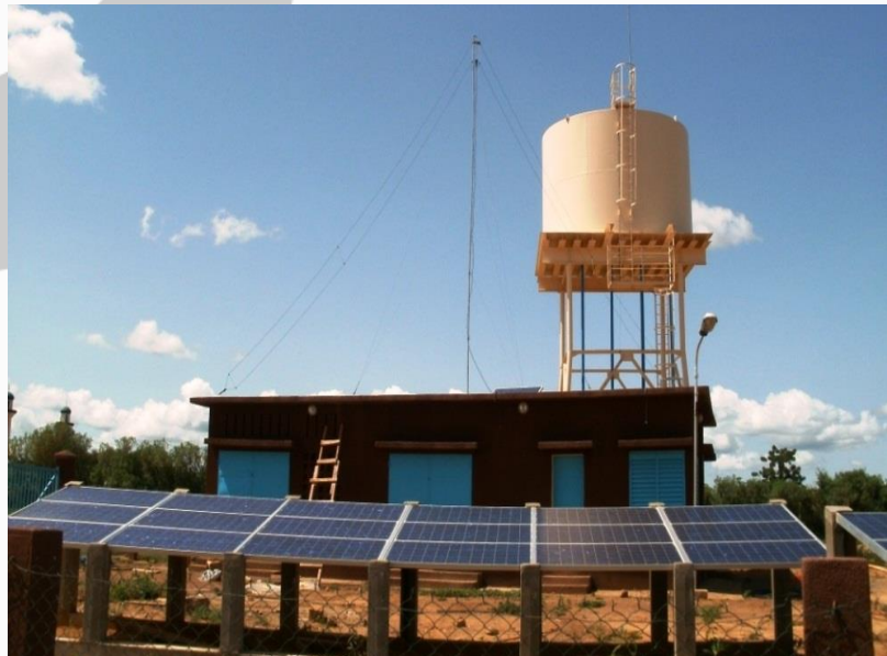
The project included the installation of 24 solar direct drive photovoltaic pumps in Mali
