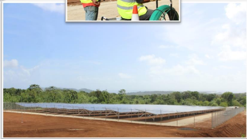
Pohnpei Photovoltaic Solutions Producing 600 kWp of Power
